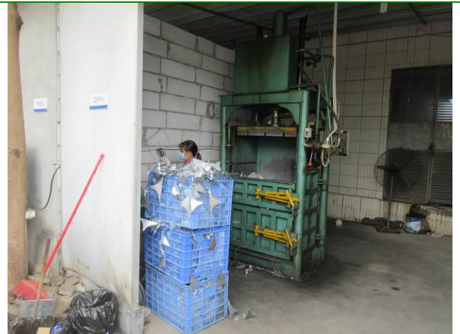
Waste treatment room
